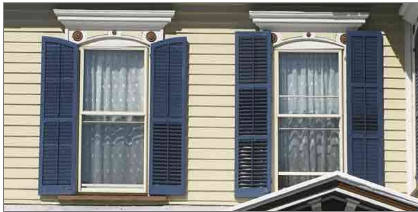
Figure 5: The shutters on the left window are appropriately shaped and sized for the related window even if they are not operable. The replacement shutters on the right are not appropriate due to the length and shape that do not correlate to the related window.
