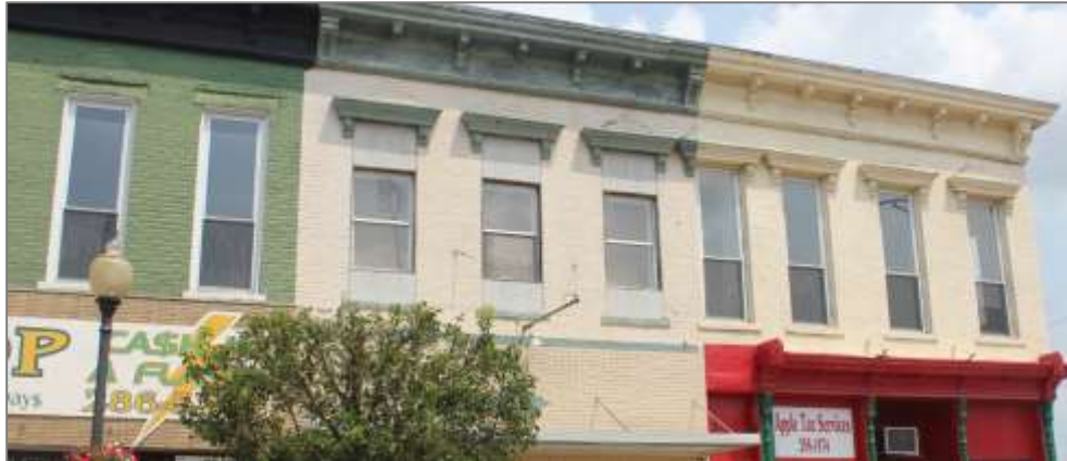
Figure 4: The window openings on the center building were inappropriately reduced in size to accommodate replacement windows that do not match the original windows in shape, size, or material.
