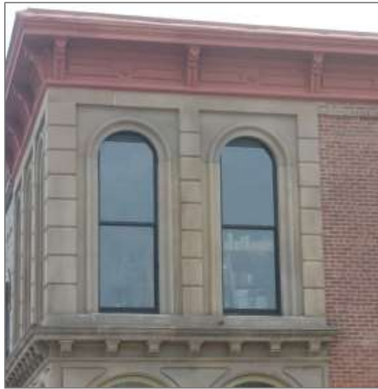
Figure 3: The above image illustrates inappropriate window replacement as the windows do not match the original window shape or design and the replacement windows are vinyl clad.
